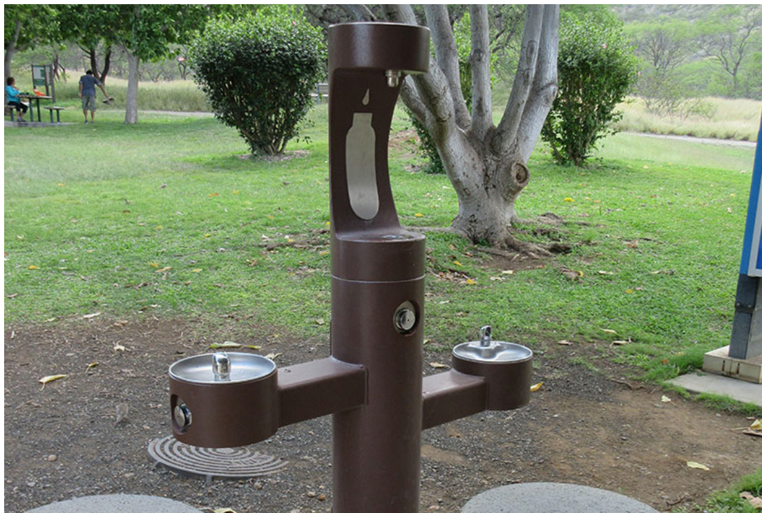
As a destination along the proposed city-wide trail system, park users and trail users alike will benefit from access to drinking fountains.
